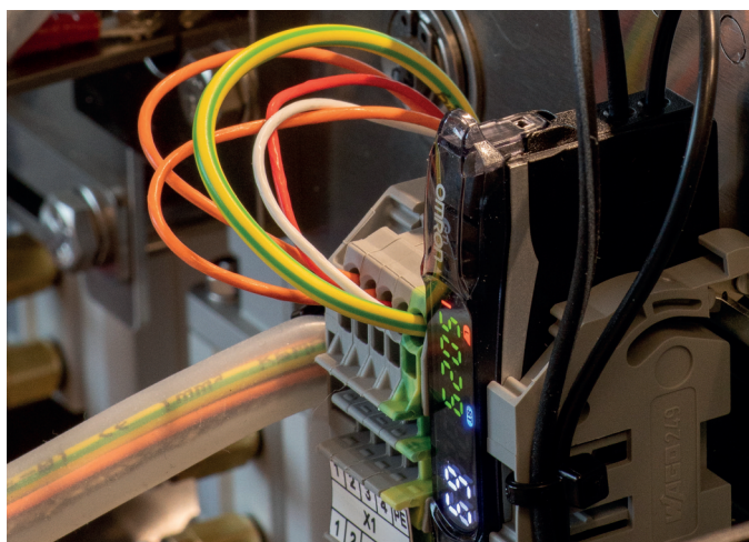
The optical sensor and fiber optic amplifier unit are linked to a programmable logic controller, allowing for seamless integration into Bandall's banding machines.
